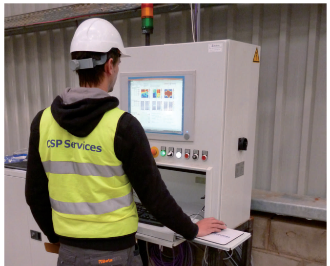
Control cabinet for automatic measurement, evaluation and output with signal light for pass or fail result
