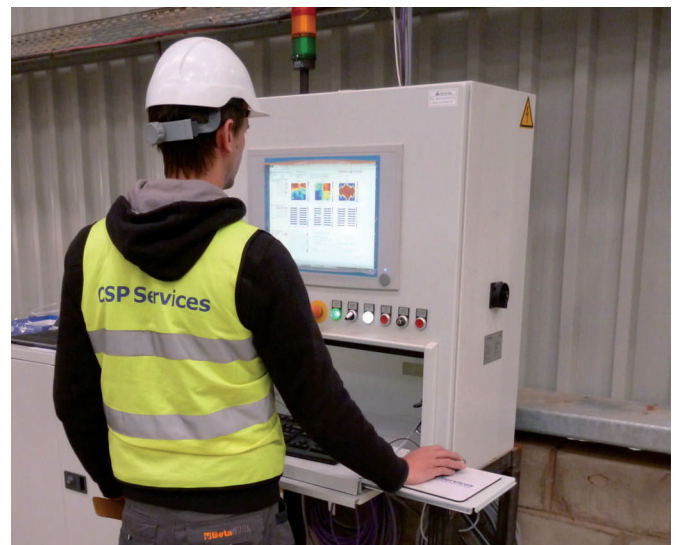
Control cabinet for automatic measurement, evaluation and output with signal light for pass or fail result
